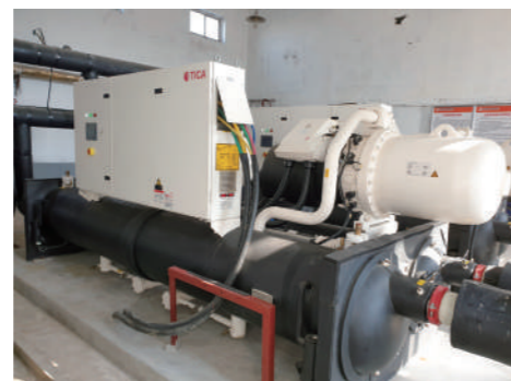
▲ Water source heat pumps
