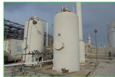
MTBE活性炭吸附罐 (LPG)
