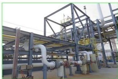
MTBE活性炭吸附罐 (PO)
